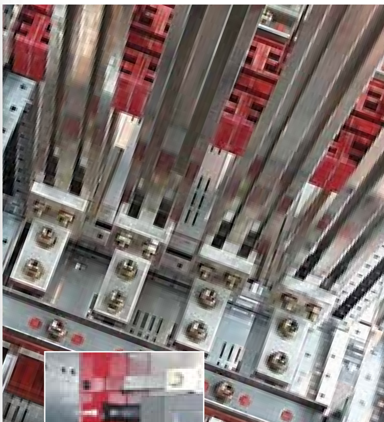
TP&N MCCB connected to distribution bars
