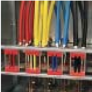
Cable connections to incoming or outgoing ACB Copperwork
