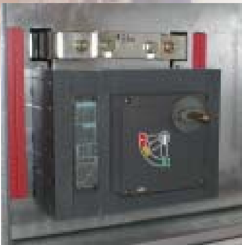
MCCB in cassette mounted in switchboard
