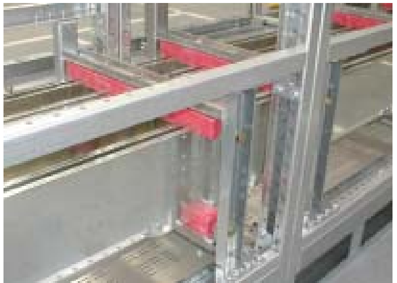
4000A main Busbars
