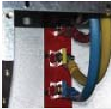
Outgoing cable connections
