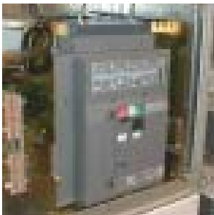
ACB housed in a 'Cassette' showing removable neutral link
