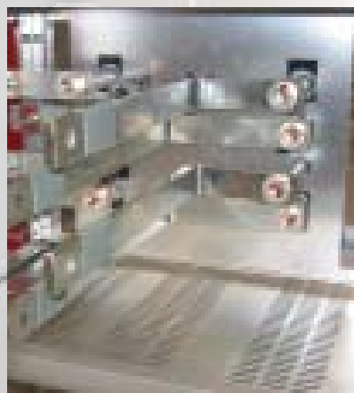
Outgoing rear connections from MCCB with insulated Busbar plate removed
