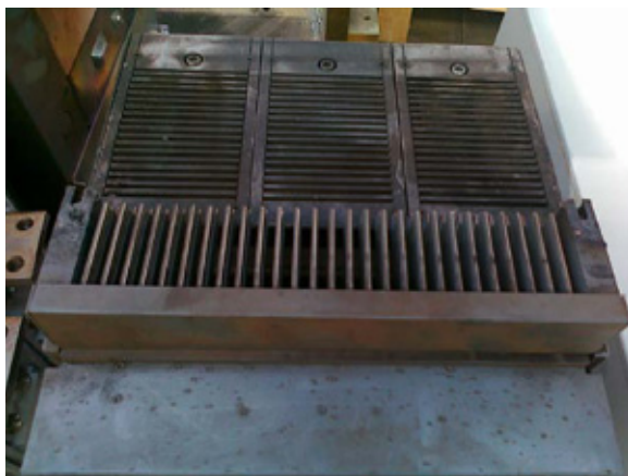
Heavy signs of short circuit current - The circuit breaker must be replaced
