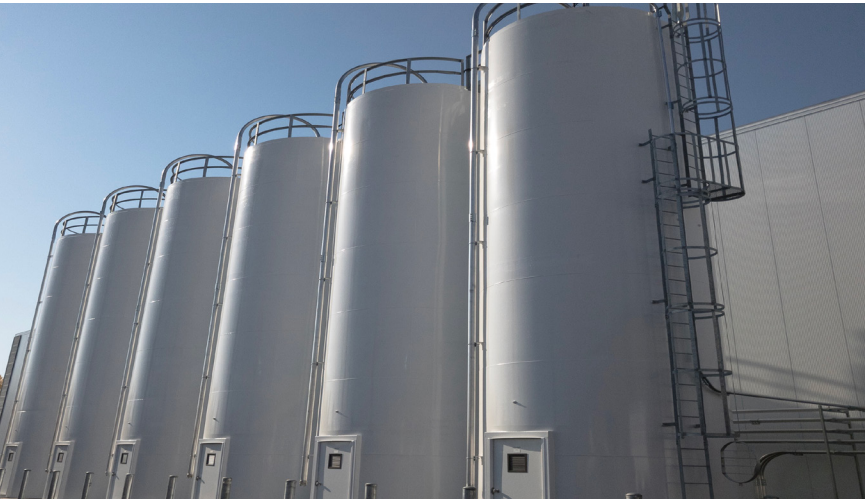
— Storage silos for plastic pellets
